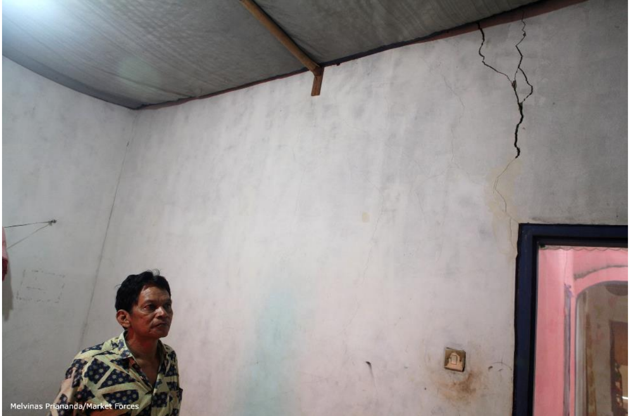
Blasting damage that occurred in 2017 at the start of Java 9 and 10 construction (2021).
